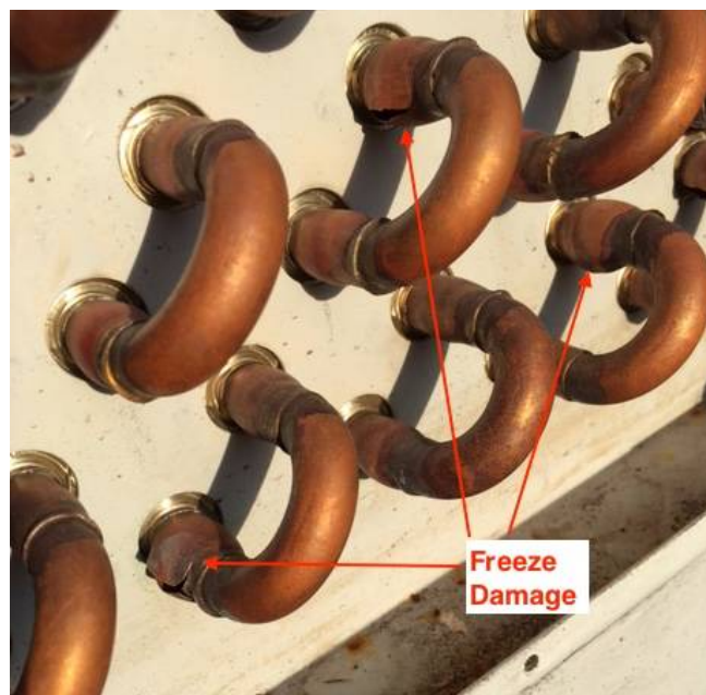
Illustration 2: Buldging and Split Tubes Caused by Freeze Damage
