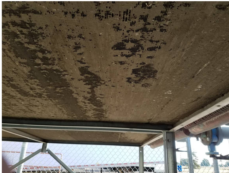
Illustration 2: Partially Blocked Heat Exchanger Coil
