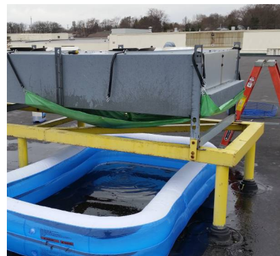
Illustration 6: Pool Beneath Air-Cooler to Capture Debris during Cleaning Process
