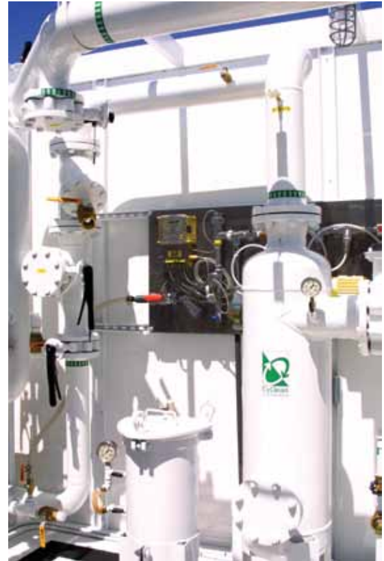
Filtration is a key factor in avoiding downtime. Shown above is a CyClean centrifugal separator with bag filter for removing dirt from an evaporative cooling tower and wall-mounted chemical feed controls to maintain water quality. Note the spare flanges on the upper left for the future installation of an additional pump to increase capacity.
